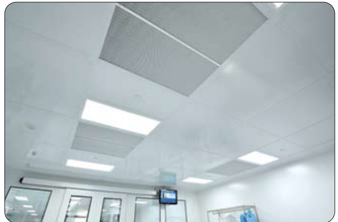
Medtronic Singapore Operations Pte Ltd (Metal Ceiling System)
