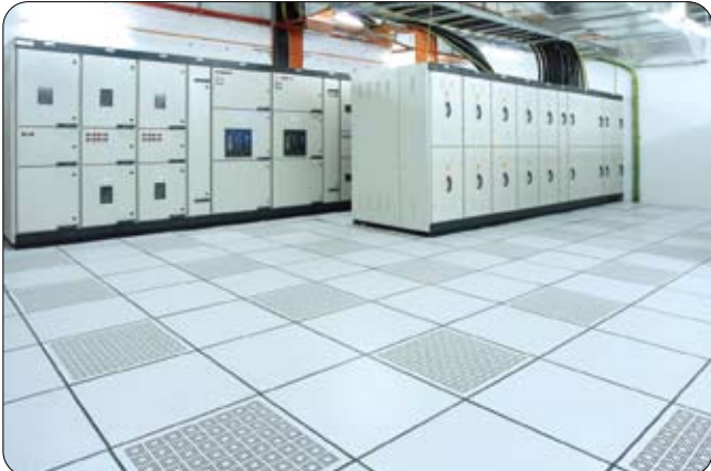
Microtac Raised Floor System installed in Control Room
