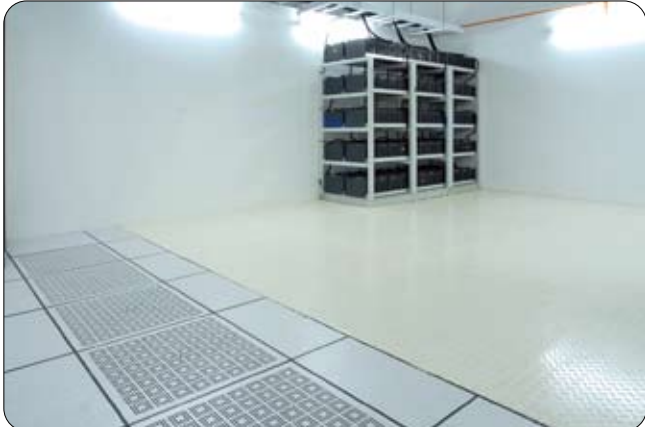
Microtac Raised Floor System installed in Battery & UPS Room
