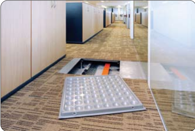
Microtac Raised Floor installed General Office
