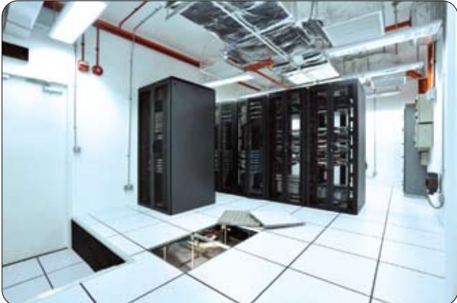
Microtac Raised Floor System installed in Server Room
