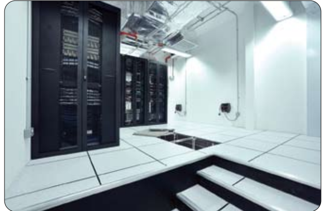
Microtac Raised Floor installed in Server Room
