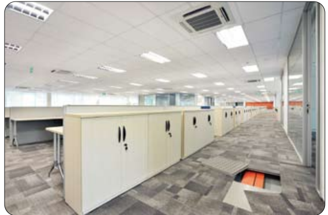
Microtac Raised Floor installed in General Office
